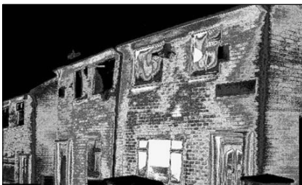
A thermal image indicating problem areas in a building.
